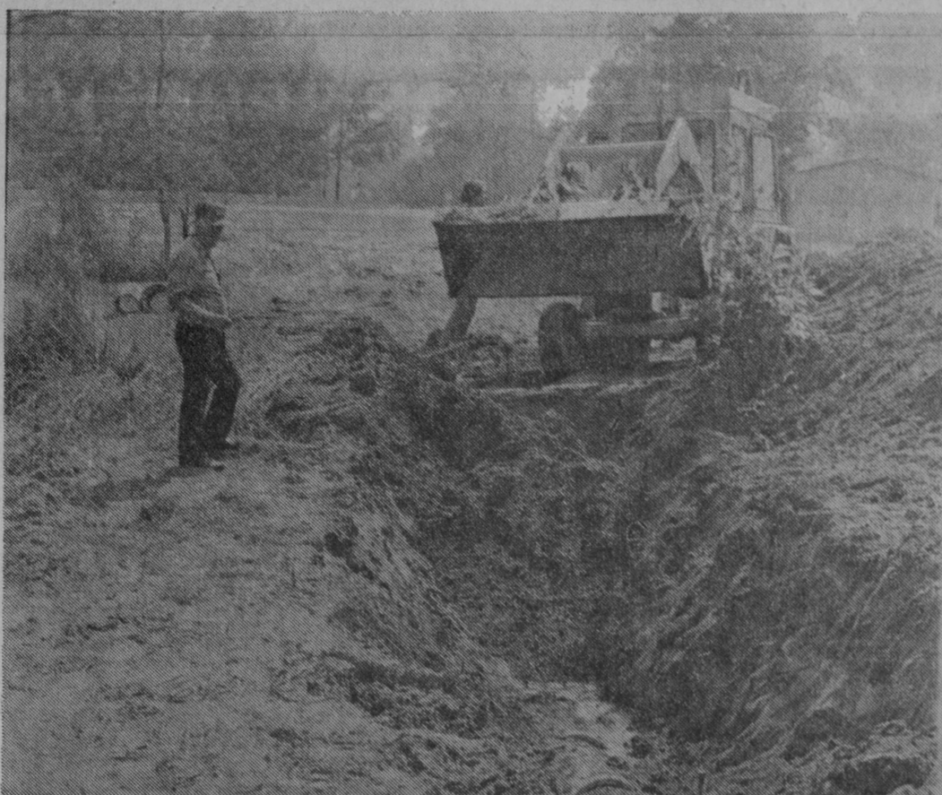
WORK WAS COMPLETED Tuesday on installation of a storm drain in the old bed of Dead Creek on city property west of the Tawas City Elementary Unit. The drain connects with a storm sewer which was constructed more than 25 years ago when the course of Dead Creek was straightened. Since then, portions of the
