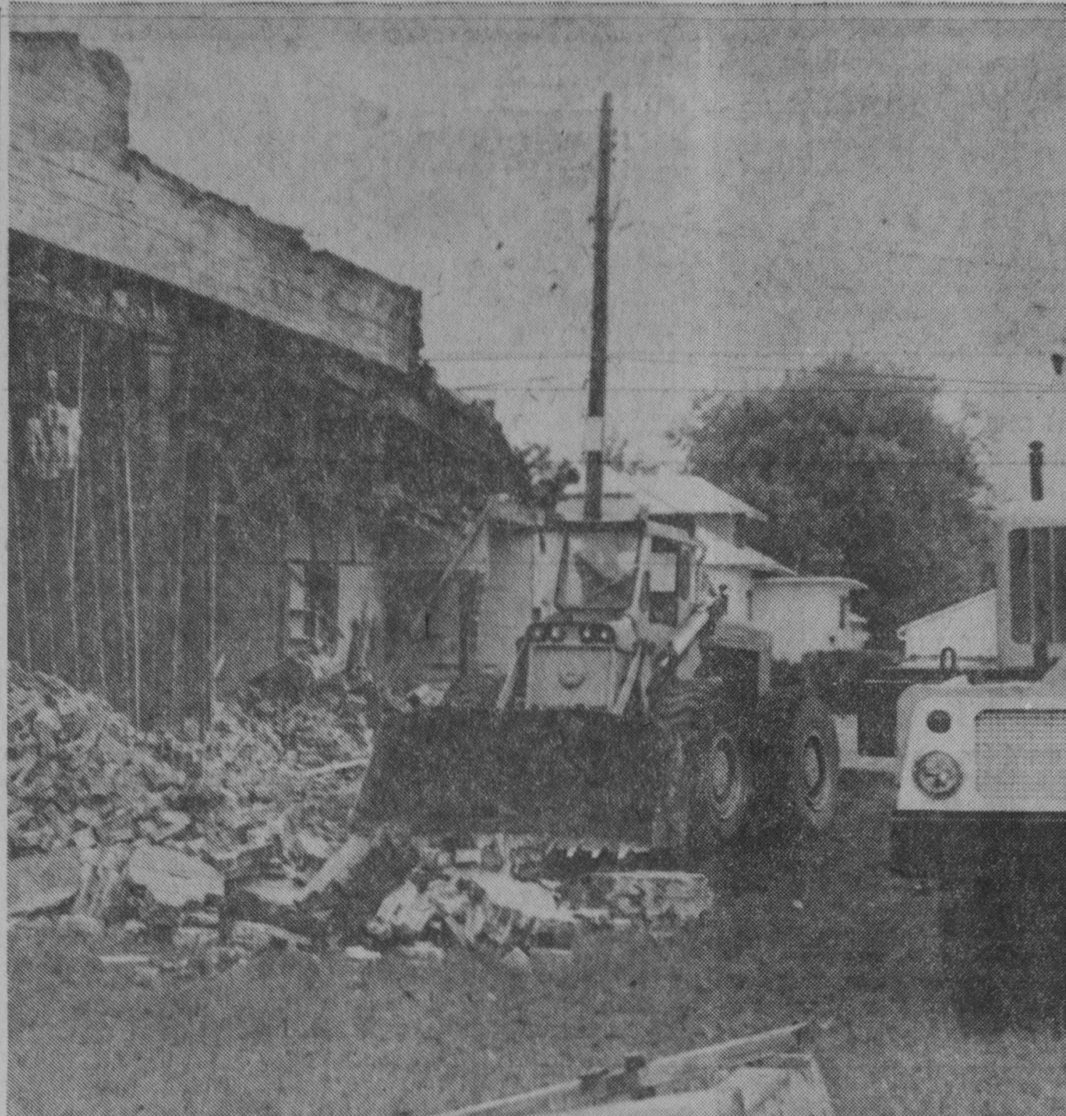
WORK STARTED MONDAY on razing the brick building which has housed Mutual Savings and Loan at East Tawas. A modern, new building is to be constructed for the firm on the site located at the southeast corner of the intersection of Newman Street and East State Street. The building was constructed on the site of the old opera house, which was destroyed by fire in the 1920s. It housed drug stores and a number of other businesses before being occupied by Mutual Savings.—Tawas Herald Photo.
