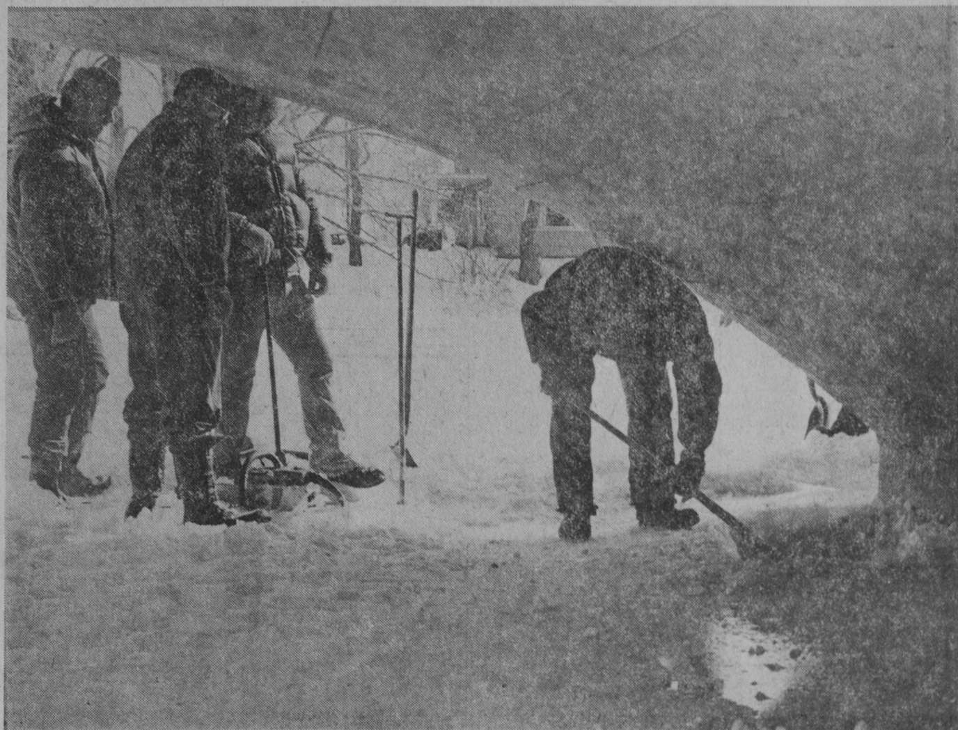
EMERGENCY REPAIRS were made to the Sixth Avenue bridge over Dead Creek last week by the Tawas City Department of Public Works. A concrete abutment on the bridge, constructed in 1912, has shown deterioration on the south end. Workmen cut
