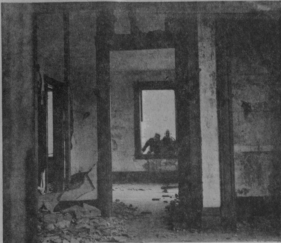
INTERIOR of the keeper's house had been ravaged by vandals when this picture was snapped. Holes were knocked in plastered walls and doors were missing. Today, the interior of the house is probably a complete shambles. —Tawas Herald Photo.
