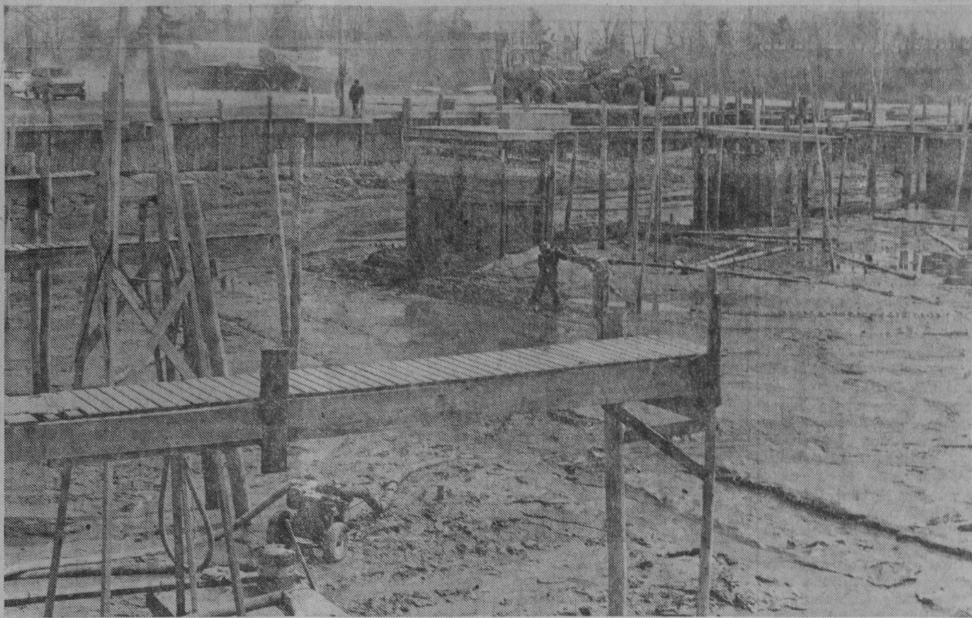
A LARGE SCALE dredging project was started earlier this spring at Tawas Bay Yacht Club on Tawas Point as members prepared for the coming boating season. With permission from the army corps of engineers, the club's boat well entrance on Tawas Bay was blocked off and water was pumped back into the
