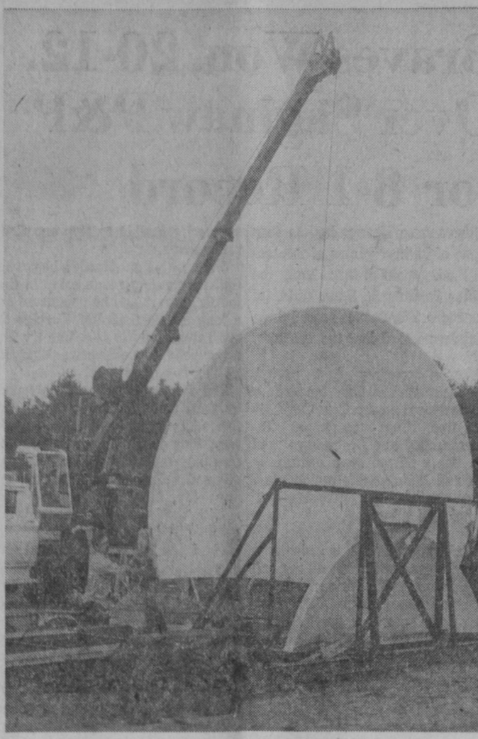
GENERAL CABLE TELEVISION began installation of its new five-meter earth station Friday at its receiver site on Kobs Road south of M-55. A Davison and Son Builders crane is being used to unload the 2,000-pound parabolic dish antenna which will be directed at a satellite 23,300 miles in space. The equipment is to be used in expansion and improvement of programming offered by the cable television firm.—Tawas Herald Photo.
