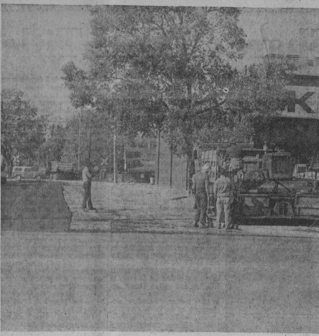
SEVERAL BLACKTOPPING PROJECTS were completed last week in Tawas City including the full width of Wheeler Street (above) west of the Kroger Store, the parking lot at the Tawas City Park, a parking strip along Eighth Avenue at the Tawas City Elementary Unit and other smaller projects. The Wheeler Street project included the parking strip next to Consumers Appliance. —Tawas Herald Photo.
