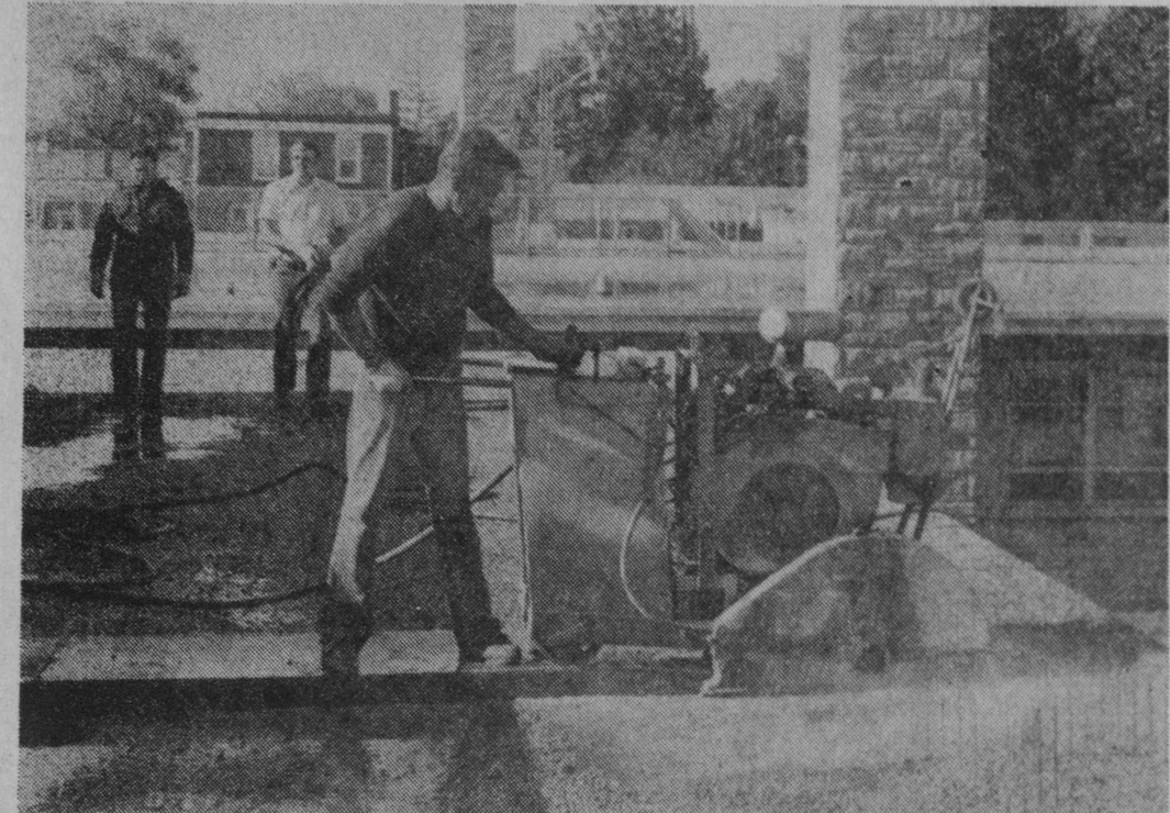
WORK STARTED Friday on cutting off an overhanging roof at the Iosco County Building in preparation for making additions and alterations
