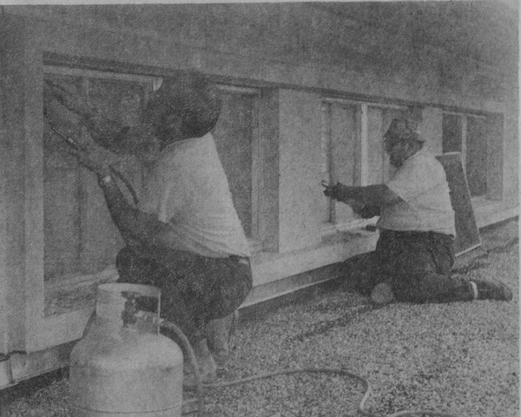
WORK STARTED Monday morning on installing 327 panes of double insulated glass in the Iosco County Building. This project is part of an energy saving program for which the county received federal funds. Charles Price and Merlin
