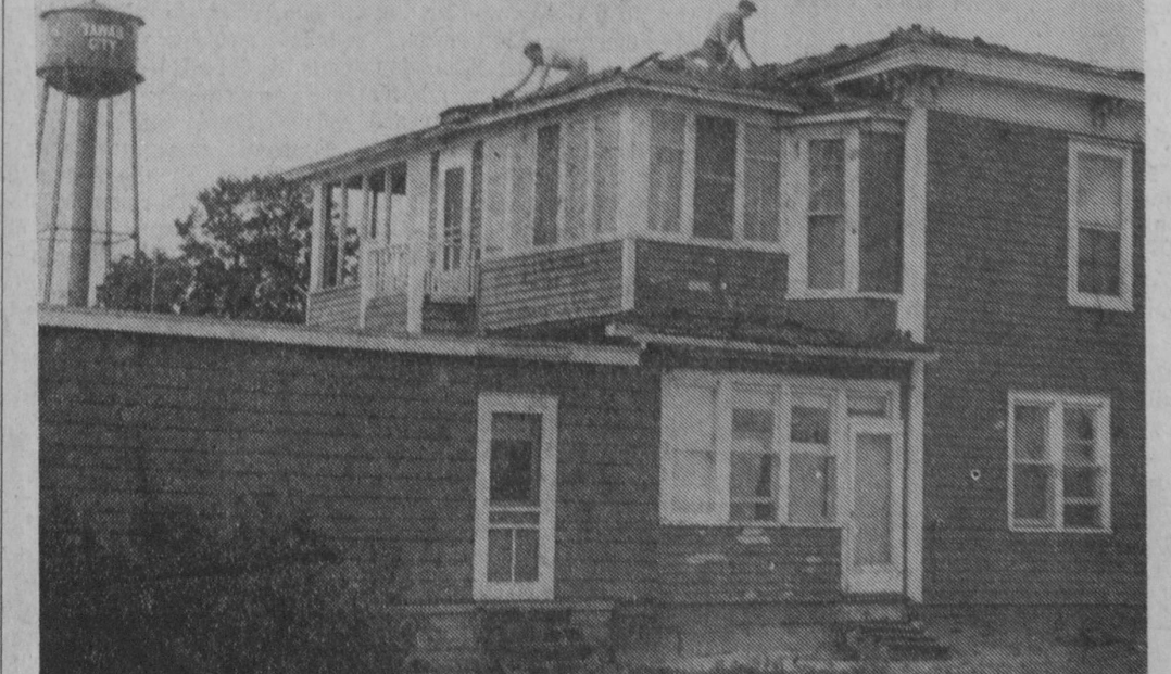
ANOTHER OLD LANDMARK in Tawas City is in the process of being razed by its owners, Carl and Brent Babcock. This house was originally constructed in the late 1870s and, after remodeling in 1884, was once the dwelling of the Nisbet family associated with the lumbering business in Tawas City. As originally constructed, a cupola was located on the roof which made a convenient spot to watch for ships entering the bay. The
