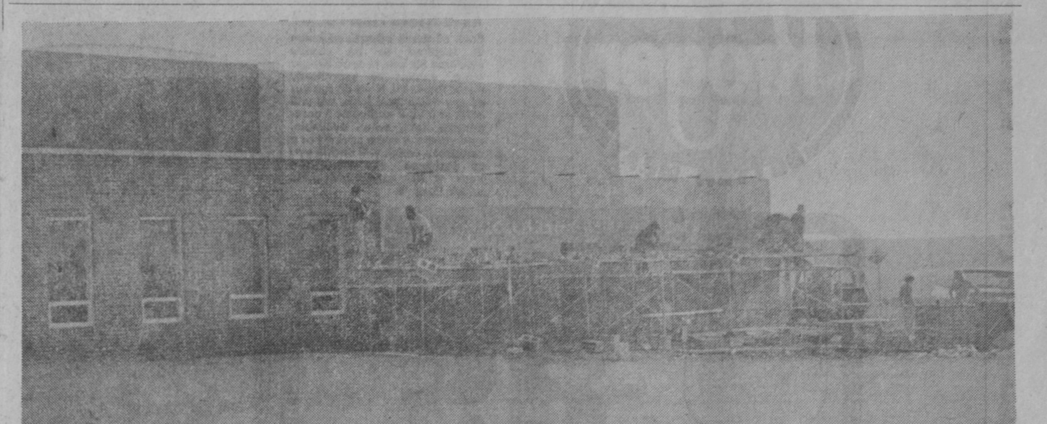
AN ADDITION to Valeron Corporation's plant at Whittemore is moving along rapidly and this picture snapped last Wednesday shows brick masons at work on the front of the structure. The 40 by 120-foot addition, to be used for heat treating and metal
