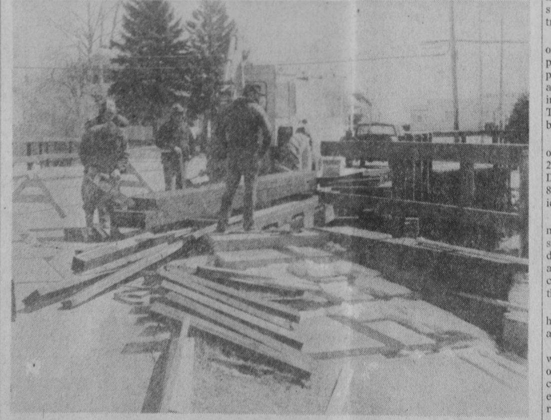
IT WAS A TOUGH WINTER on bridges in Tawas City. Work started Tuesday by the department of public works on making repairs to the Mathews Street bridge, which was damaged months ago when an automobile went out of control and crashed into the railing. Temporary repairs were made earlier to the Whittemore Street bridge which was damaged by an automobile.—Tawas Herald Photo.
