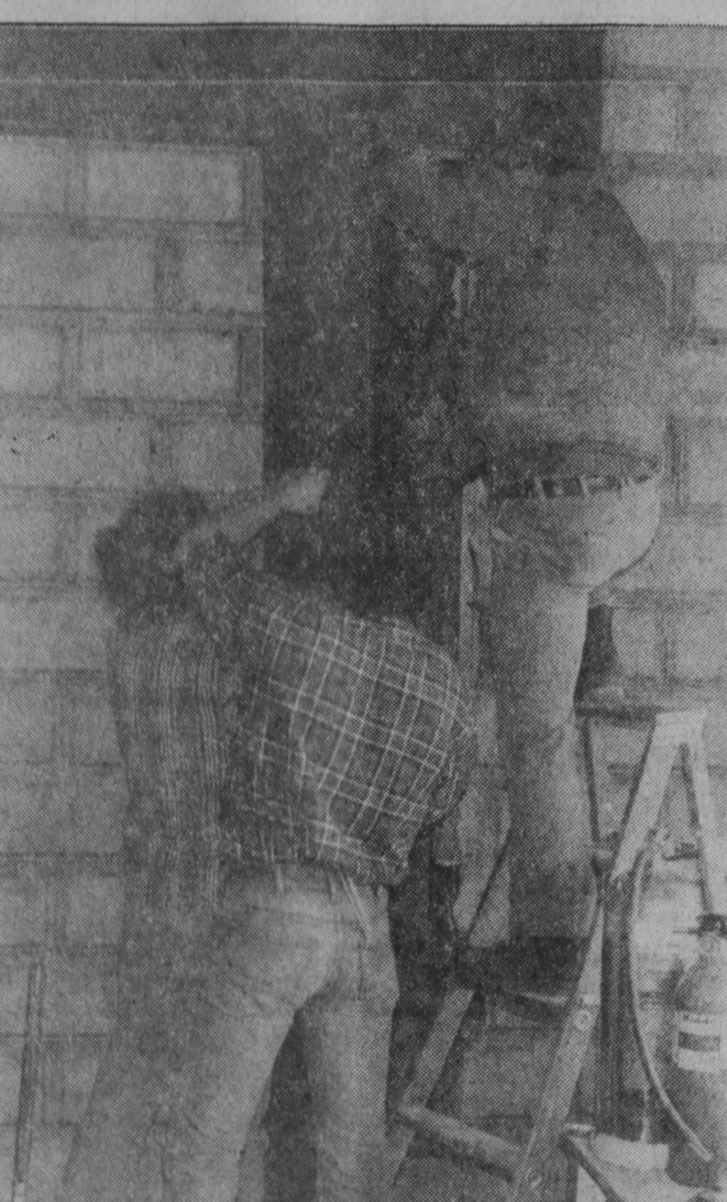
WORK STARTED last week on enlargement of Kelsor's Econo-Way Drug Store in Tawas City. The new floor plan will utilize both the present drug store and the former variety store.
