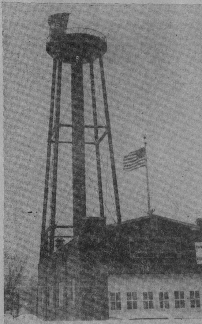
ANOTHER STEP in the removal of a Tawas City landmark was witnessed Wednesday when Urban Wrecking Company completed removal of the bowl of the Tawas City water tank. After cutting the tank into strips, the last piece was removed Wednesday. Remainder of the 42-year-old tower structure will be razed in the days ahead.—Tawas Herald Photo.
