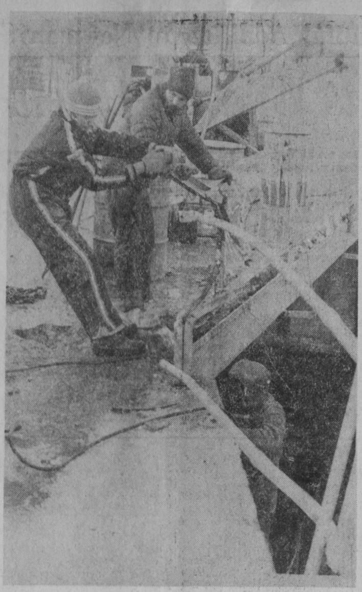
TEMPORARY REPAIRS were made last week to the Whittemore Street Bridge in Tawas City. The old bridge was knocked out of commission several weeks ago when a car crashed into a railing. The structure was damaged to such an extent that it was blocked off to traffic. Members of the city crew welded a steel girder back into position and repaired the railing.—Tawas Herald Photo.
