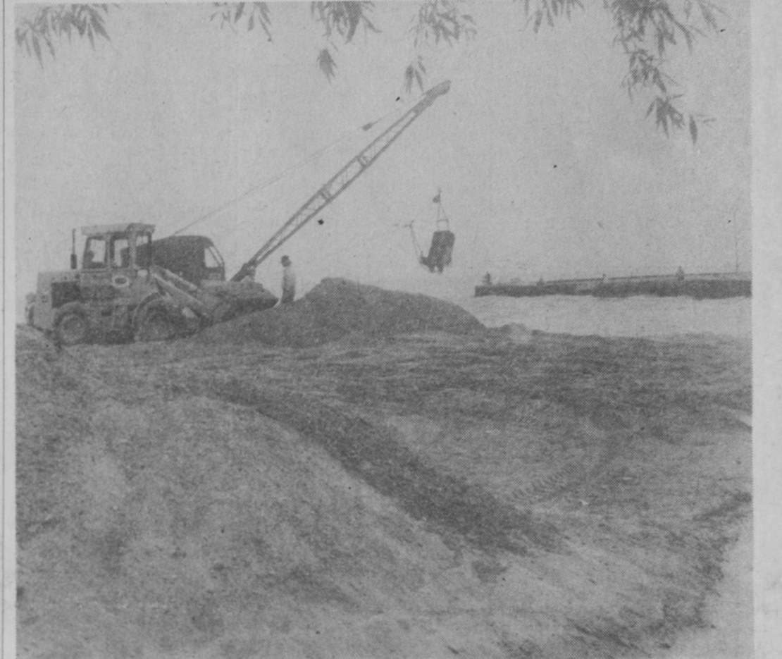
A CONTINUING PROCESS—Equipment of the Tawas City Department of Public Works swung into action Friday to open the mouth of the Tawas River, which had become partially clogged in recent weeks by shifting sand. Sand removed from the river bottom was used to fill an old
