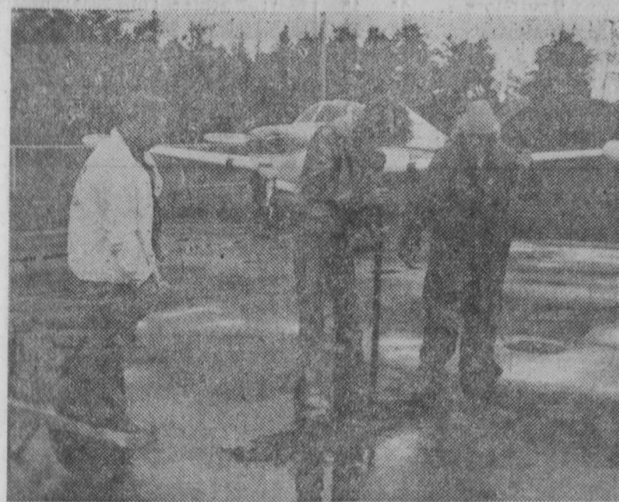
PATCHING runways, mending fences and general maintenance provides employment for three public service employment participants on a Comprehensive Employment Training Act (CETA) program at the Isosco County Airport. Richard Backus, left, supervises Steven Dodd and Ralph Daubenspeck in a maintenance project. This CETA program and many others in Isosco County are funded through Region 7B Employment and Training Consortium, Harrison.
