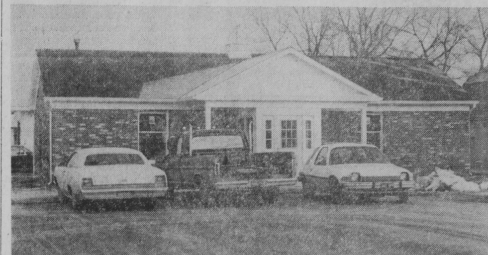
PROGRESS on the new Hale branch office of Peoples State Bank of East Tawas is pictured above as of Wednesday. Contractor for the project is Davison and Son Builders, Tawas City. The new office is located at the northeast intersection of M-65 and Esmond Road.—Tawas Herald Photo.
