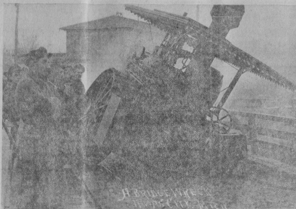
LIFE of the Mathews Street bridge was shortened when this heavy steam traction engine plunged through its oak deck. The man at left is Rudolph Stark, who had charge of removing the steam engine and making repairs to the bridge.
