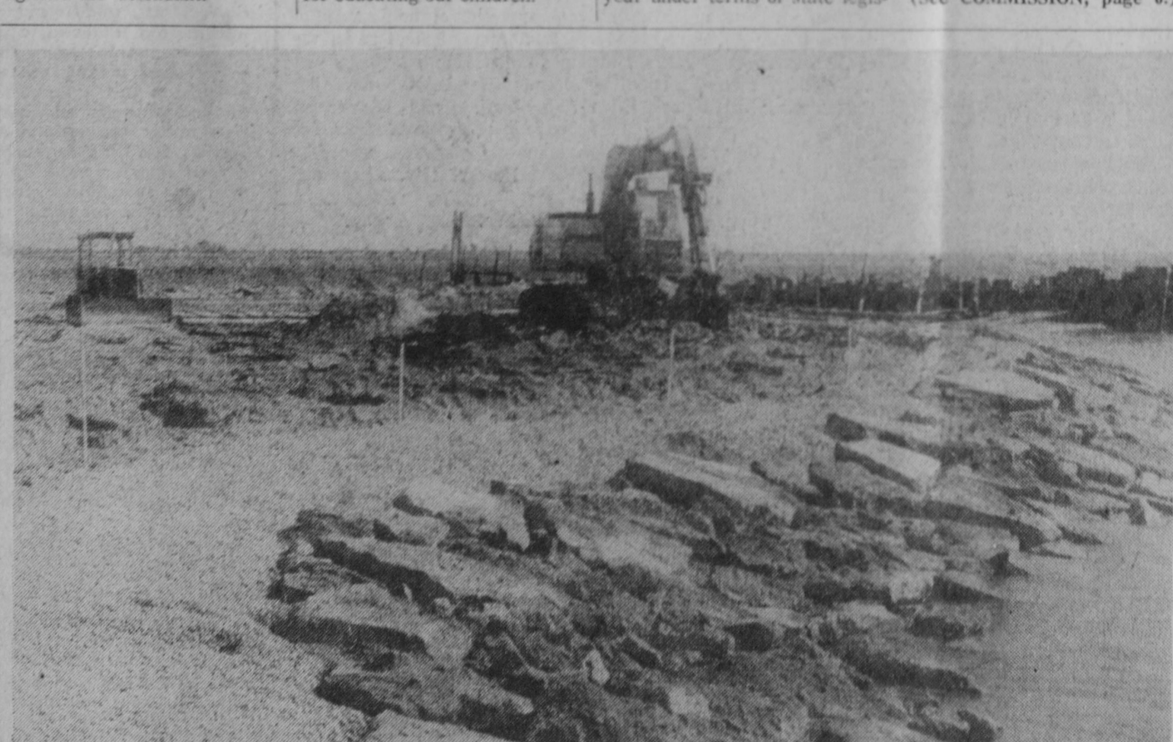
WORK started last week on an earth filled groin to protect the new state boat launching ramp at East Tawas. This structure is being constructed in Tawas Bay at the former site of the Captain Mac pier east of the state police post. Work is expected to be completed this fall on concrete ramps for the boat launching area, with onshore facilities to be constructed next spring. Room for this new facility came through the recent demolition of the former East Tawas City Garage west of Hester's Market. The groin is to protect boats from wave action while being launched in the bay.—Tawas Herald Photo.
