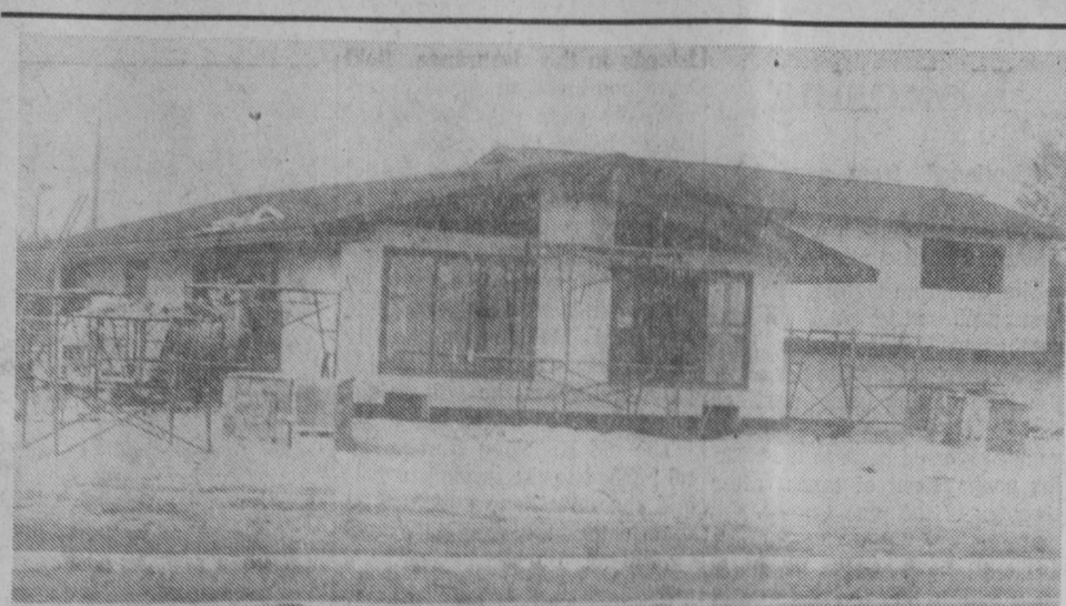
WORK is progressing so rapidly on the new parish house of Immaculate Heart of Mary Church that any picture snapped seems to be outdated by the time it is published. This picture was snapped last week, but stone masons were busy later in the week constructing a fireplace chimney and changed the entire exterior appearance of the building. The beautiful new building is located on the site of the former school overlooking Tawas Bay and fronting on Lake Street in Tawas City.—Tawas Herald Photo.
