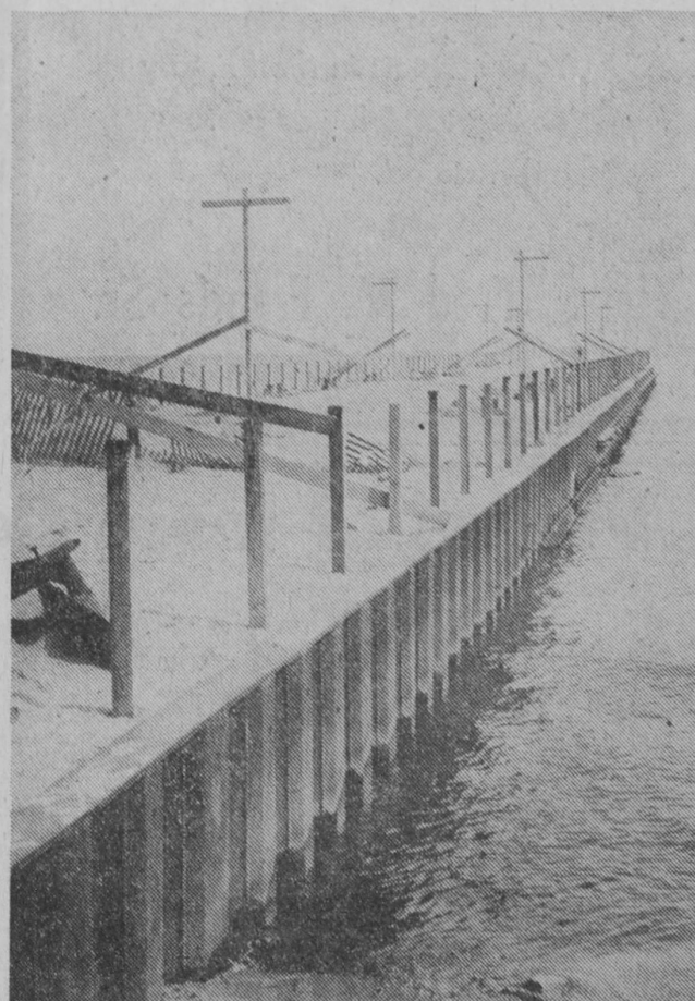
PROGRESS on the final phase of reconstruction of the fishing pier at the Tawas City Park is shown here. A wooden railing has been constructed along the dock, with support posts for a new lighting system. The project, financed through a cooperative program between the state and city, is to include two blacktop sidewalks along the outer edge of the dock, benches and picnic tables.—Tawas Herald Photo.
