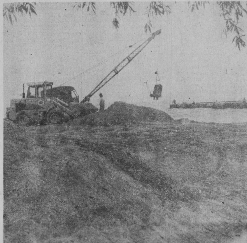
FOLLOWING PURCHASE of the east side of the river mouth, the City of Tawas City began filling in a boat slip, using sand removed
