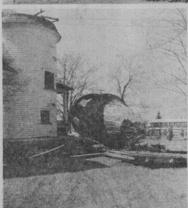
THE TWO VIEWS show the start of demolition of the old school building in 1957. A chain has been attached to the belfry and it is about to be yanked to the ground in the top picture, pausing for an instant before making its final plunge. Wreckage is shown in the lower view.—Tawas Herald Photos.
