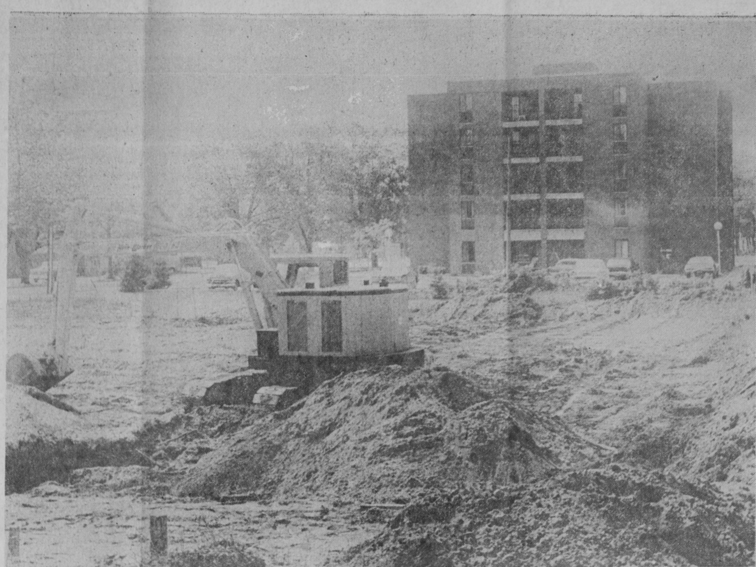
CLEARING the site for the new Bay Park Tower-North has been completed and work is under way on digging foundations for the five-story apartment building for elderly housing. After long months of struggling, the East Tawas Housing Commission headed by John C. Elliott was able to cut through bureaucratic red tape to sell 1.650-million dollars
