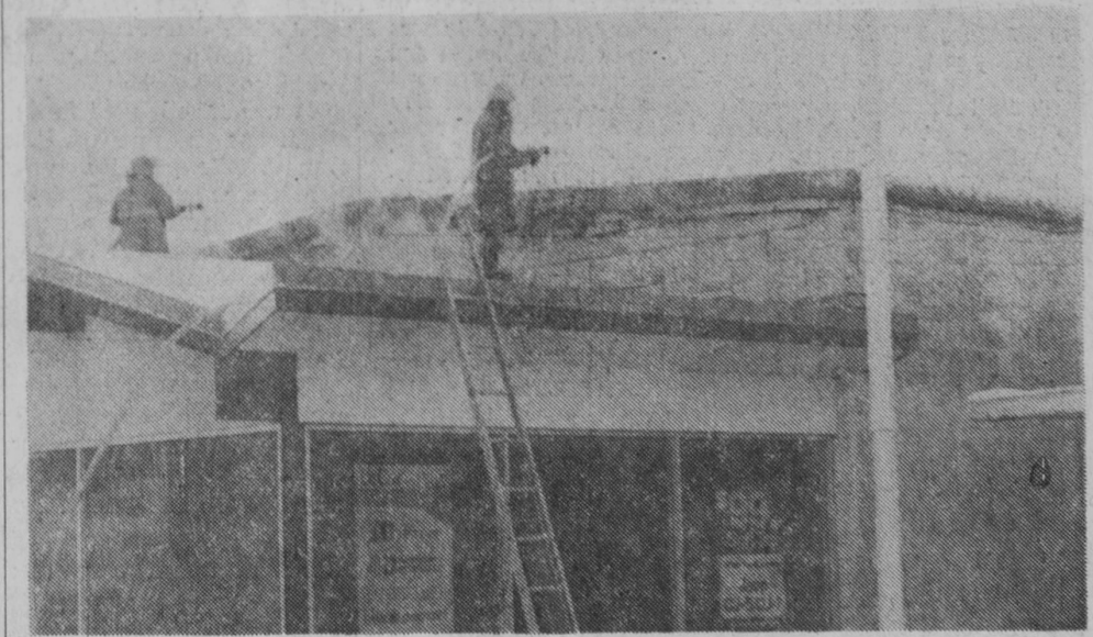
TWO FIREMEN stand on the roof of the salesroom of Barbier Motor Sales and pour water through the burning roof of the garage portion. The blaze started in a parts room and a wall helped to contain the flames.—Tawas Herald Photo.
