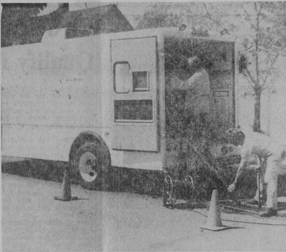
A TELEVISION CREW is at work this week at East Tawas, but the "production" is not expected to reach network presentation. Actually, the crew is making a television survey of sewer mains in the city to perform maintenance work and also to look for places where ground water seeps into the mains as part of an area wide grant from federal-state funds to upgrade waste treatment facilities.—Tawas Herald Photo.
