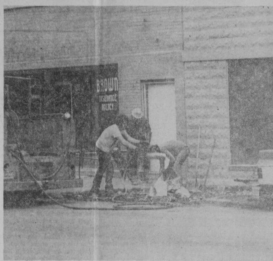
A COOPERATIVE construction program with property owners in replacing damaged sidewalks was started last week by the City of Tawas City. One of the first projects was replacement of sidewalk on the east side of Whittemore Street, using the city's crew. The picture above shows damaged sidewalk being removed from in front of Huron Auto Parts. James Fowler was con-
