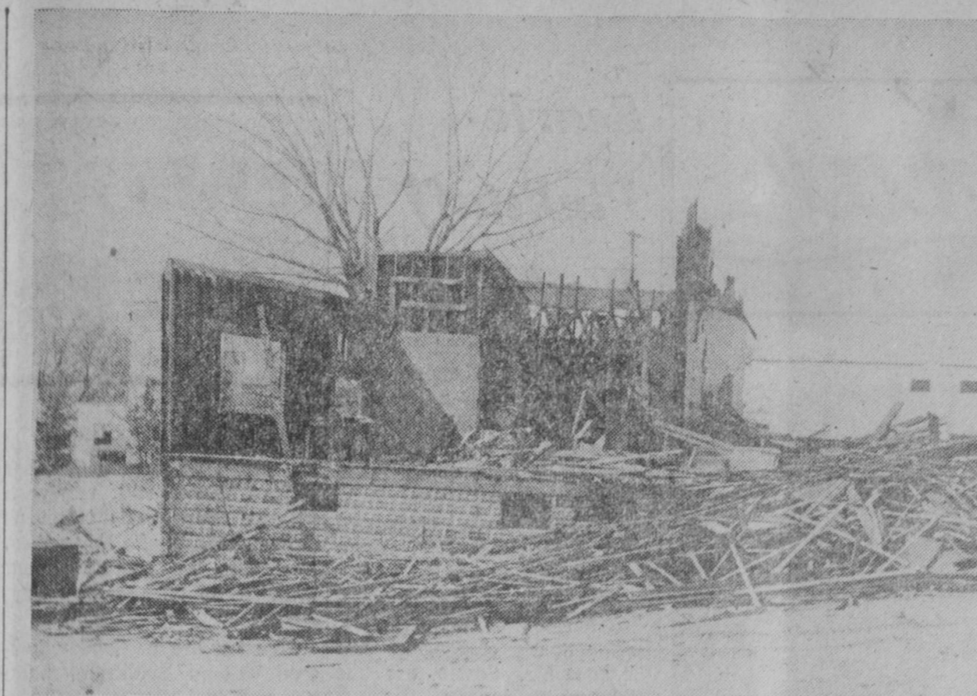
PROGRESS on demolition of this old building on Lake Street, Tawas City, is shown as of Tuesday morning. At Monday night's city council meeting, Coun. Donald Hayes proposed that the city adopt an ordinance to control demolition of buildings to insure removal during a specified time period. —Tawas Herald Photo.
