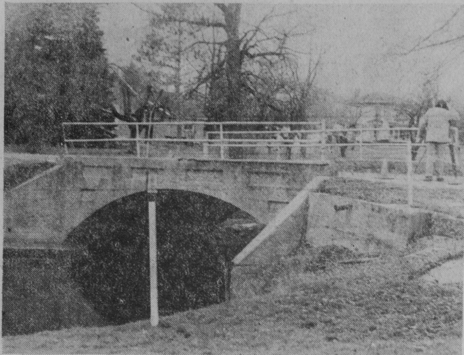
AN EMPLOYEE of Edmands Engineering Company of Bay City is shown taking elevations at the Sixth Avenue bridge over Dead Creek Tuesday afternoon in preparation for removal of the structure starting today (Wednesday). The bridge is to be replaced by a two-span wooden structure. —Tawas Herald Photo.
