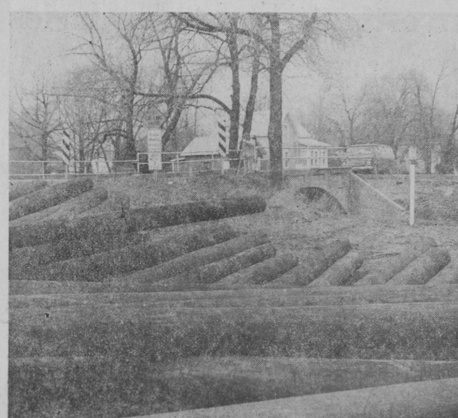
WOODEN PILING for the new bridge over Dead Creek at Sixth Avenue arrived Tuesday morning and Great Lakes Contractors of Warren is scheduled to start removal of the bridge today (Wednesday). The new wooden span is to replace a concrete bridge constructed by C. H. Fowler in 1912.—Tawas Herald Photo.
