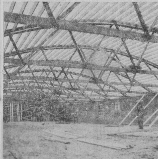
THIS PICTURE was snapped in 1950 while the building was under construction by James Boomer of Tawas City. The project was finished two weeks ahead of schedule.
