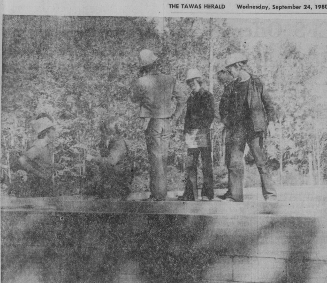
BUILDING TRADES CLASSES of Tawas Area High School are now working on constructing a new house on Victoria Lane, Tawas City, as an annual project of the vocational training program. Wet weather has delayed progress at the start of the school term and Lucky Kosto, instructor, has been working short handed while Robert Reasner, veteran building trades instructor, has been recuperating from an ankle injury.—Tawas Herald Photo.
