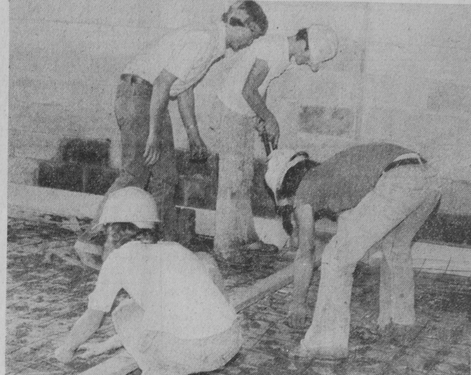
DAVID LUTZ, left, supervises CETA trainees as they prepare to make the last pour of concrete at the Grant Township Fire Hall. Turn to page 2, sec. 2, for more pictures.—Tawas Herald Photo.
