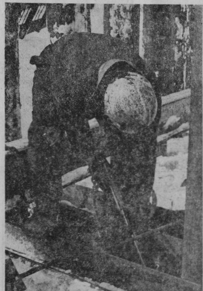
THIS WORKMAN is using a cutting torch to prepare steel beams being used to straighten the piling for the Whittemore Street bridge. A dam built across the river downstream from the bridge to collect debris has raised the river about 18 inches at the bridge site and has slowed the flow of the river. As a result, the ice forming on the river has provided a convenient "platform" for workmen.—Tawas Herald Photo.
