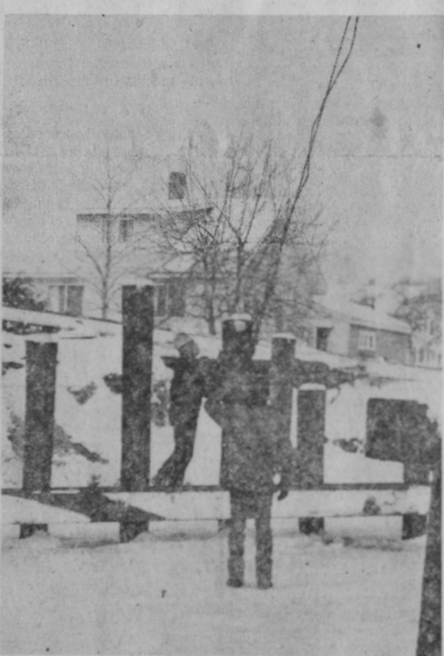
THESE MEN are attaching a long cable from a dragline in preparation to straighten the wooden piling. The treated piling was driven 25 feet into the river bottom and some veered off course after striking a solid object—possibly rock—below the stream bed. The posts will be cut off later to a uniform level for installation of wooden beams to form the bed of the roadway.—Tawas Herald Photo.
