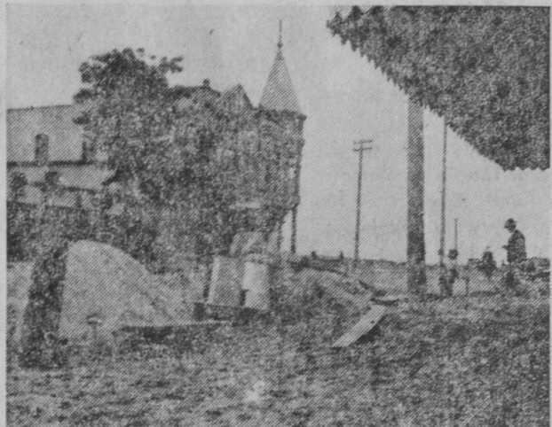
BOARD SIDEWALKS were being replaced when this view was snapped shortly before 1965. Workmen are constructing a sewer line along the west side of the street.
