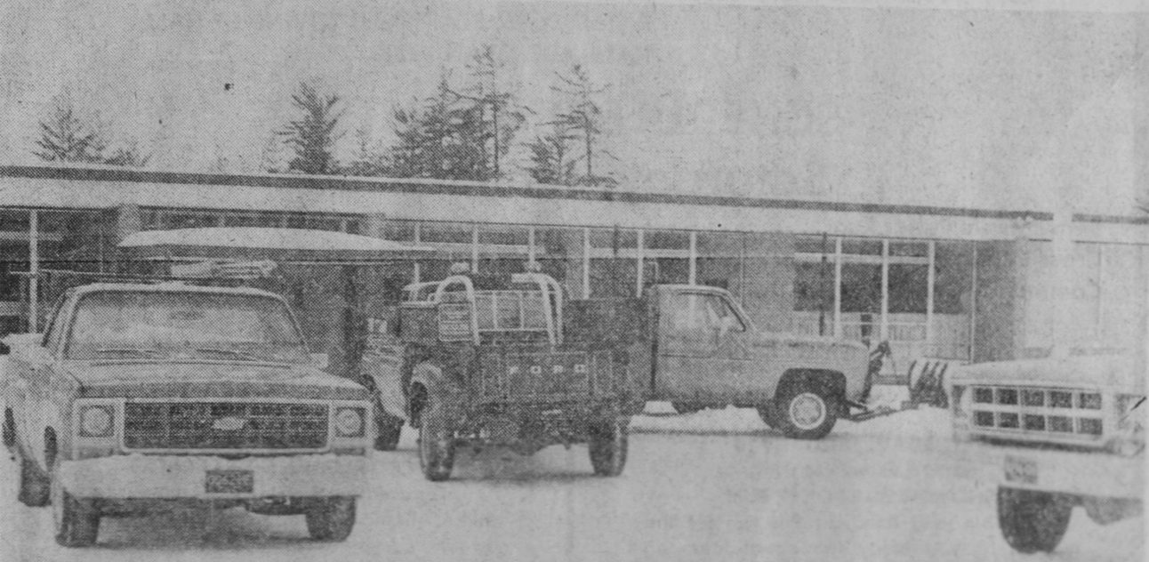
A CREW of men worked 24 straight hours to make repairs to Tawas Area High School's heating system which was damaged Saturday night by freezing weather. The bottom picture shows a lineup of trucks Monday morning in front of the school.—Tawas Herald Photos.
