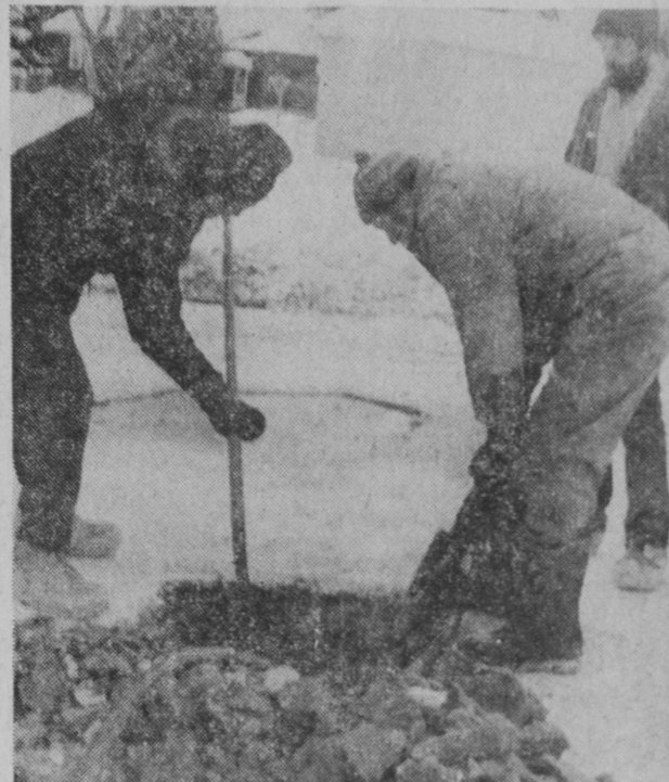
AN AIR HAMMER was used Monday morning by the Tawas City Department of Public Works crew to dig a hole in Harris Avenue in order to locate and repair a broken water main.—Tawas Herald Photo.
